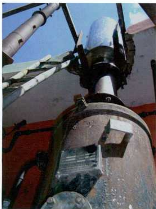
Figure 4: Ushma Shoshak unit fitted on the 100 kg capacity boiler
