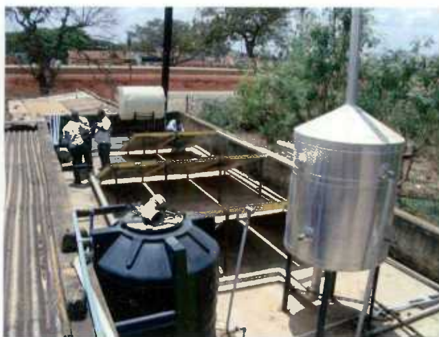
Figure 3: 600 l additional insulated tank with 1000 LPD solar water heating system installed on the roof of multiend silk reeling unit
