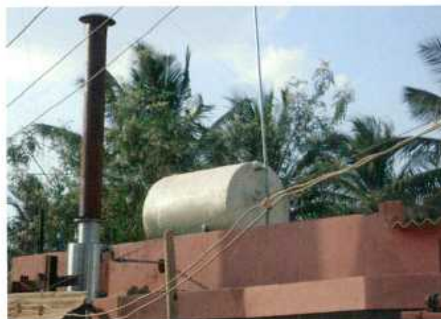
Figure 2: 600 l additional insulated tank and Ushma Shoshak unit fitted to the boiler chimney passage
